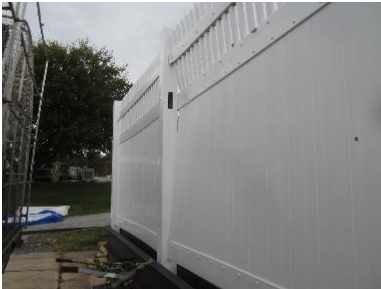
Photo No. 3 Fence Failure / Configuration 1b - Tremont
